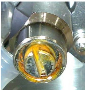
Figure 4 The trace of corrosion on the drain valve after running the chiller with C6F14 and C6.
